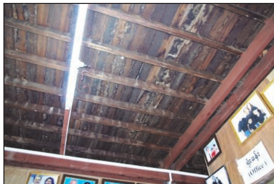
We need ceiling tiles between the 1st and 2nd floor
