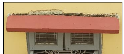
Poor condition of the walls and windows
