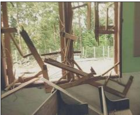
Bomb damage to a church in Khamphat Village
