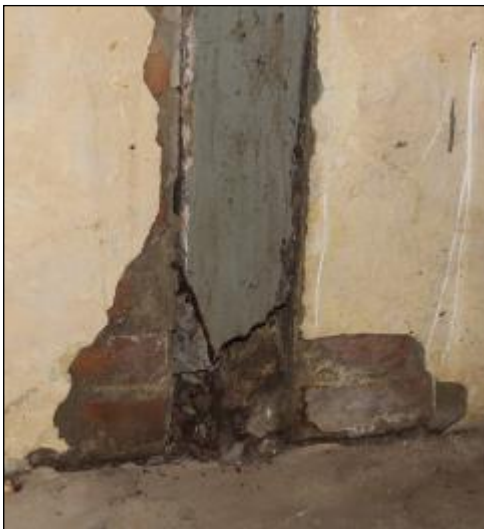
The foundation is crumbling.
